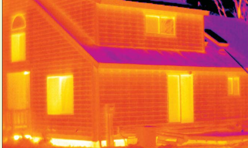
Ever wonder where your dollars go? For this family, through the windows, eaves, and a very poorly insulated roof. Thermal image courtesy FLIR Systems, Inc.
